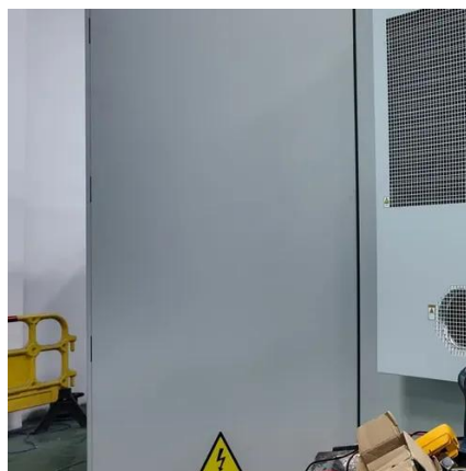
Energy storage container, BESS container
