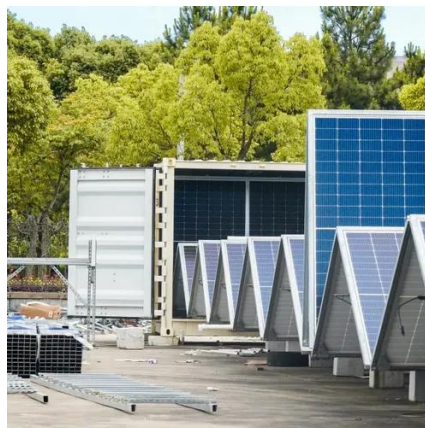
Energy storage container, BESS container
