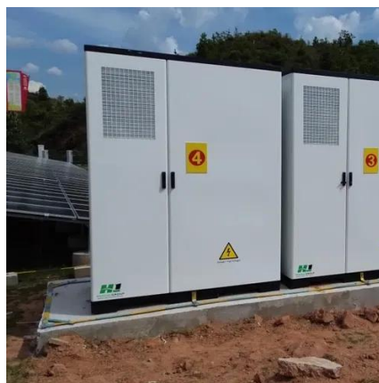
Containerized energy storage , Microgreen.ca
