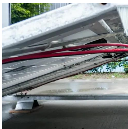
Energy storage container, BESS container
