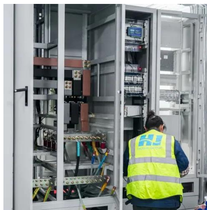
Electrical breaker panel in mozambique
