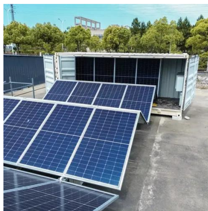
Containerized energy storage , Microgreen.ca
