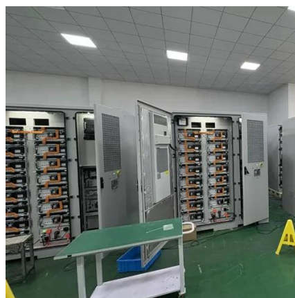
Huawei Tunisia Energy Storage Industrial Project
