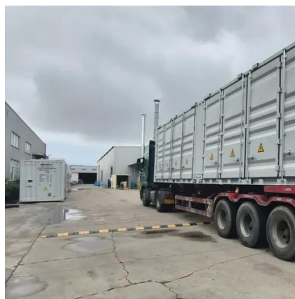
Containerized energy storage , Microgreen.ca
