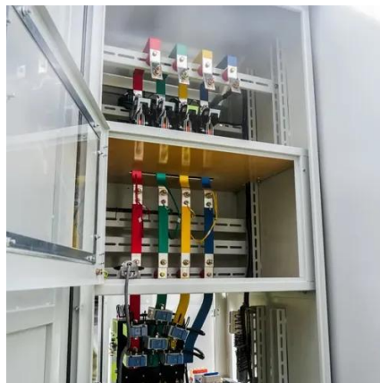
Containerized energy storage . Microgreen.ca
