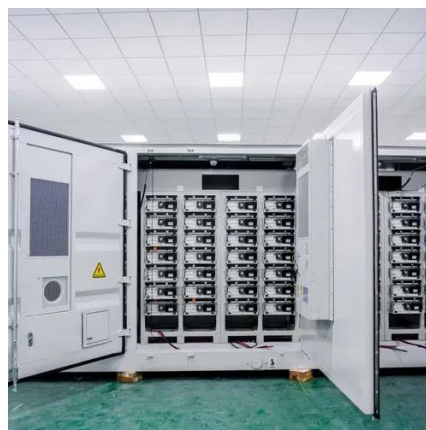
Battery energy storage system (BESS) container, ...
